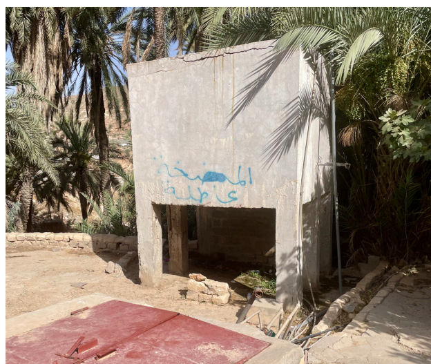
Figure 2. A Broken Water Well in the Jabal Nafusa.
